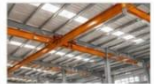
LIGHT CRANE SYSTEMS
