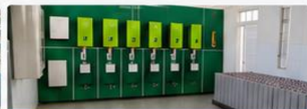
AHQ HOSPITAL LANDIKOTAL (132 KW) HYBRID SYSTEM WITH BACKUP – YEAR 2018
