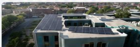
ROOF MOUNT STRUCTURE APS Warsak Road – (45.6 KW) – YEAR 2020
